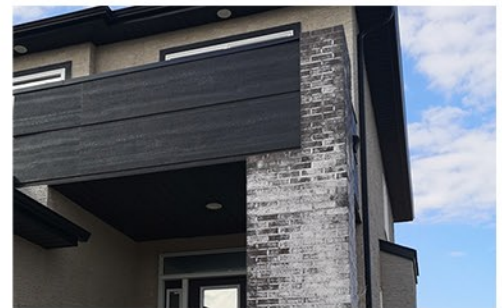
Black brick with efflorescence staining on the face from repeated water exposure.
